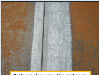
Blasted surface area, this particular model is fast and efficient in the removal of coatings, paint and rust.
